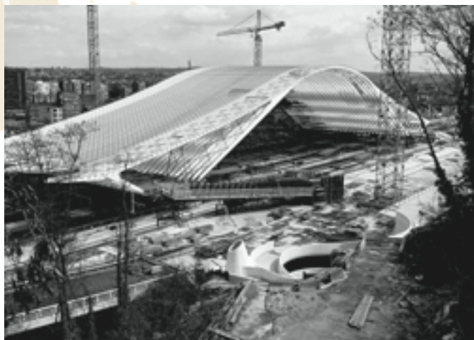
The new rail station in Liège, designed by Santiago Calatrava, under construction.
